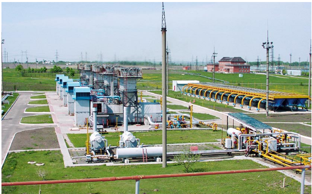
Compressor unit of a gas pipeline at Kursk, Russia. Source: S. Lechtenböhmer, Wuppertal Institute
