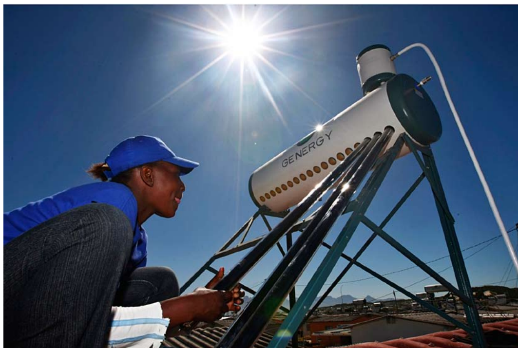
Installation of a solar-thermal facility as part of CDM Project 0079 in Kuyasa, South Africa.
